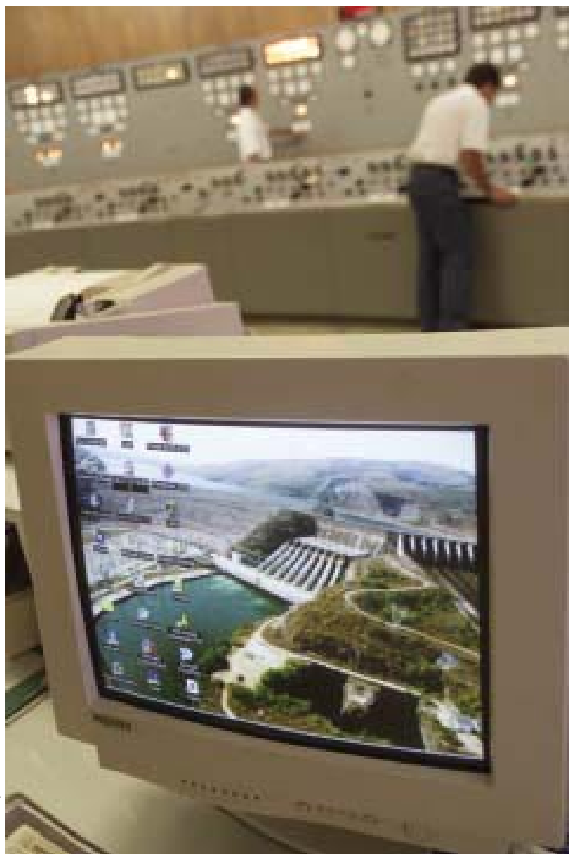
Control room of the Furnas Hydroelectric Power Station (State of Minas Gerais)
